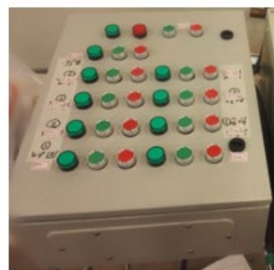
(f) Control board
