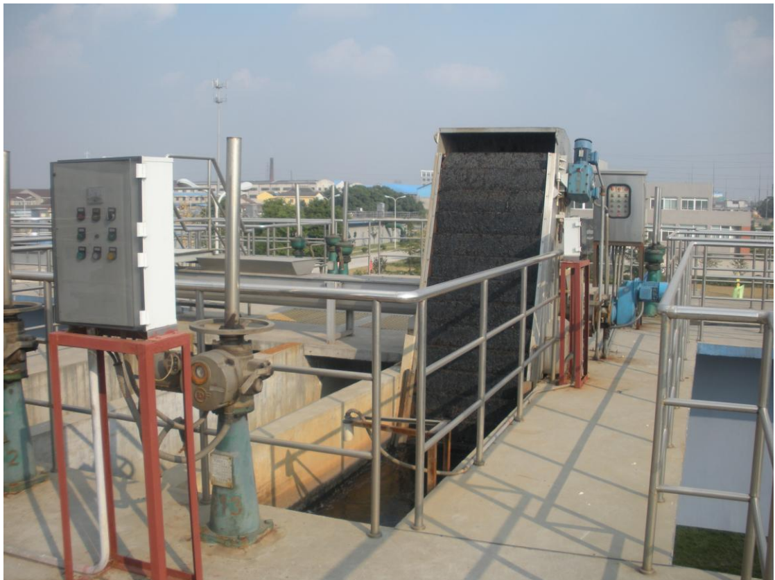
Figure 3.3 Fine screen before the vortex grit-water separation tank
