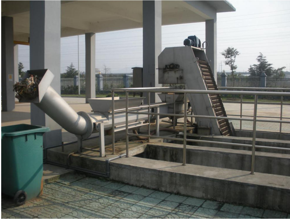
Figure 3.2 Primary lifting pumps with coarse grid
