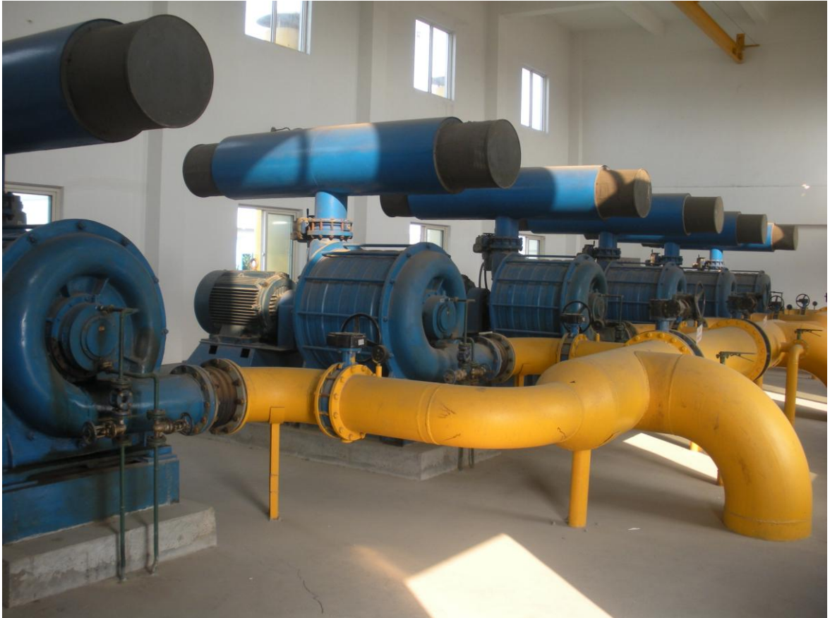
Figure 3.7 Six blowers in the air blaster system
