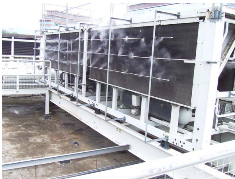
Figure 4.2 A photo of the studied chiller
