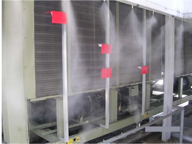
Figure 5.6 Photograph of the water mist system with data loggers
