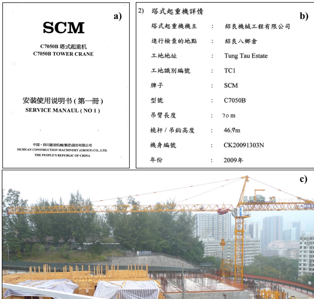
Figure 4.6 An example of tower crane information: a) service manual of tower crane; b) detailed information of tower crane; c) tower crane in the construction site
