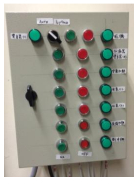
(e) Control board
