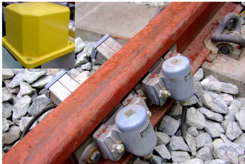
Figure 17. Electronic axle counter formed by two pairs of transmitter and receiver installed in a rail closely. The inset exhibits converter equipment connecting the axle counter at the trackside.
