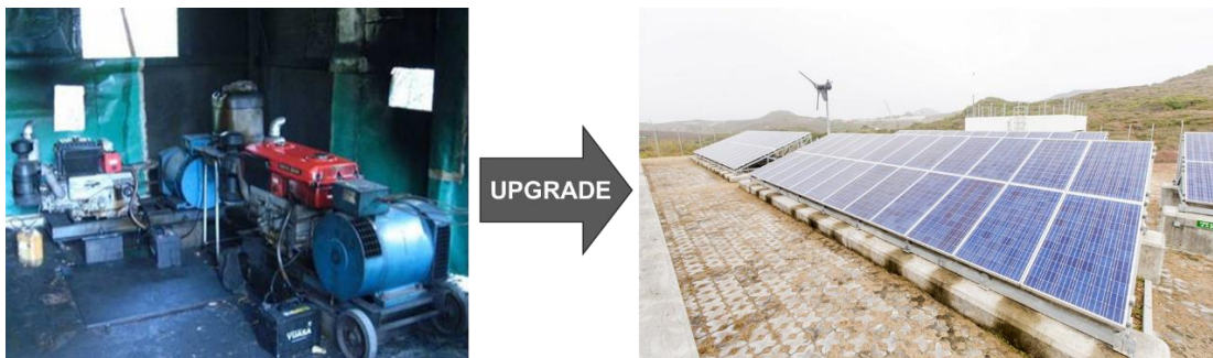
Figure 2-1 – Diesel generator used to power Town Island before system upgrade (left) (CLP, 2010) and Town Island Microgrid (right) (CLP, 2019)
