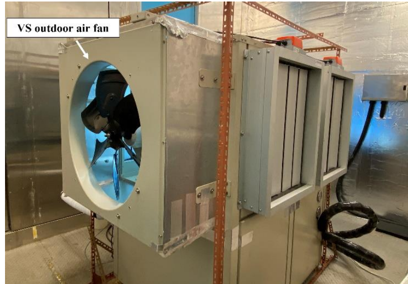
Photo 1 The VS outdoor air fan of the experimental VS ASHP unit
