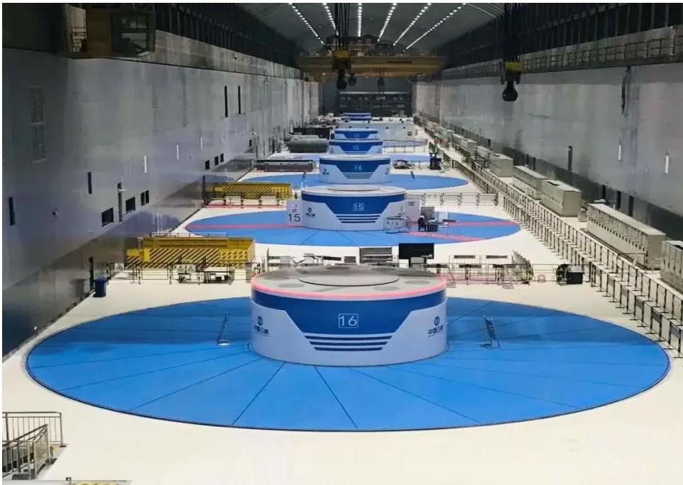
(b) The 16 units of Baihetan Hydropower Station
