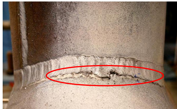
Failure mode: punching shear
