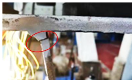
b) Typical fatigue crack of WTR
