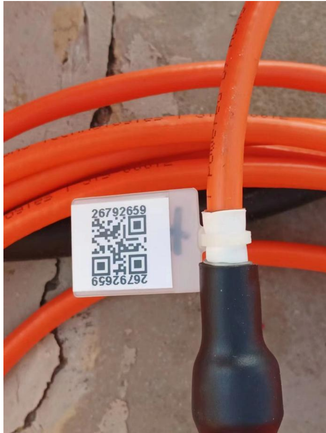
Figure 3-22 LumiCon sensor probe (black) and cable (orange)
