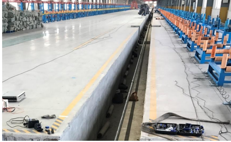
Figure 5.2 Photograph of the cable
