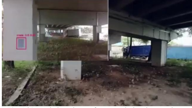
Fig. 5.21 Crack detection performance during the experiment.
