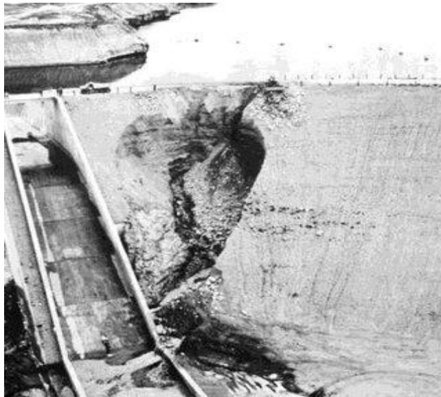
Fig 1.2 Piping failure on the right abutment of Fontenelle Dam in Wyoming, USA, in 1965 (Babu and Srivastava 2014).
