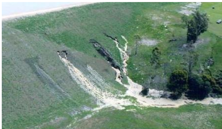
Fig 1.3 Failure of the Tunbridge Dam due to internal erosion in Tasmania, Australia, in 2008 (Yousefpour and Mojtahedi 2024).
