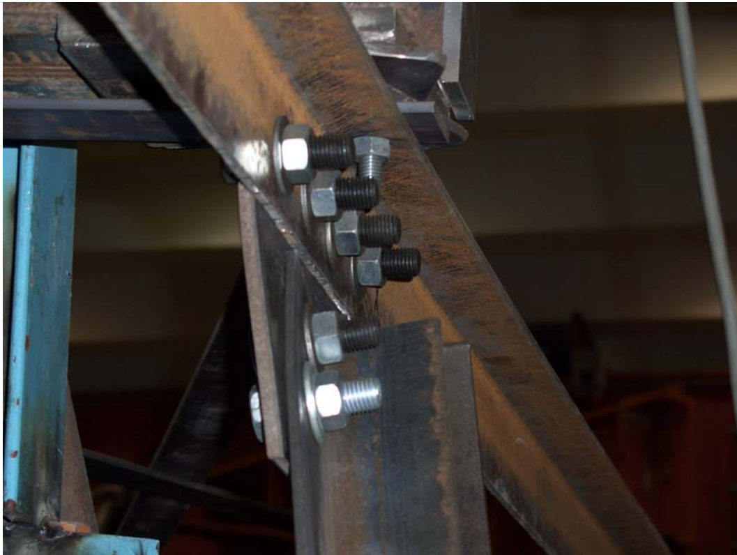
Figure 7.8 Rotation of the specimen at the connection (webs on same side, double-bolted)
