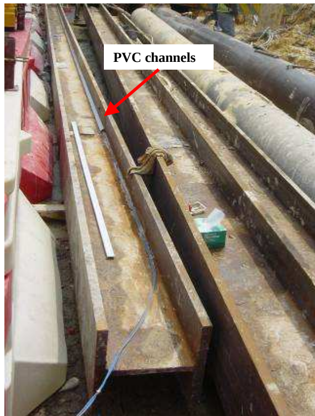
(c) Protection of optical fiber cables by PVC channels
