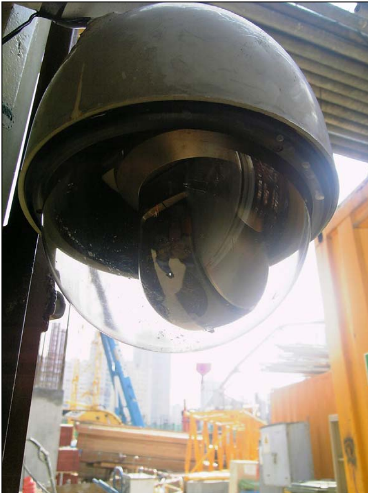
Figure 13. Network camera inside a dome housing
