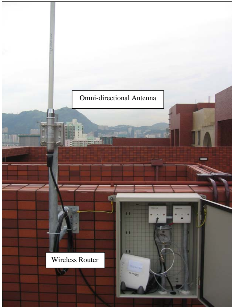
Figure 19. An omni-directional antenna and a wireless router connected to the Internet
