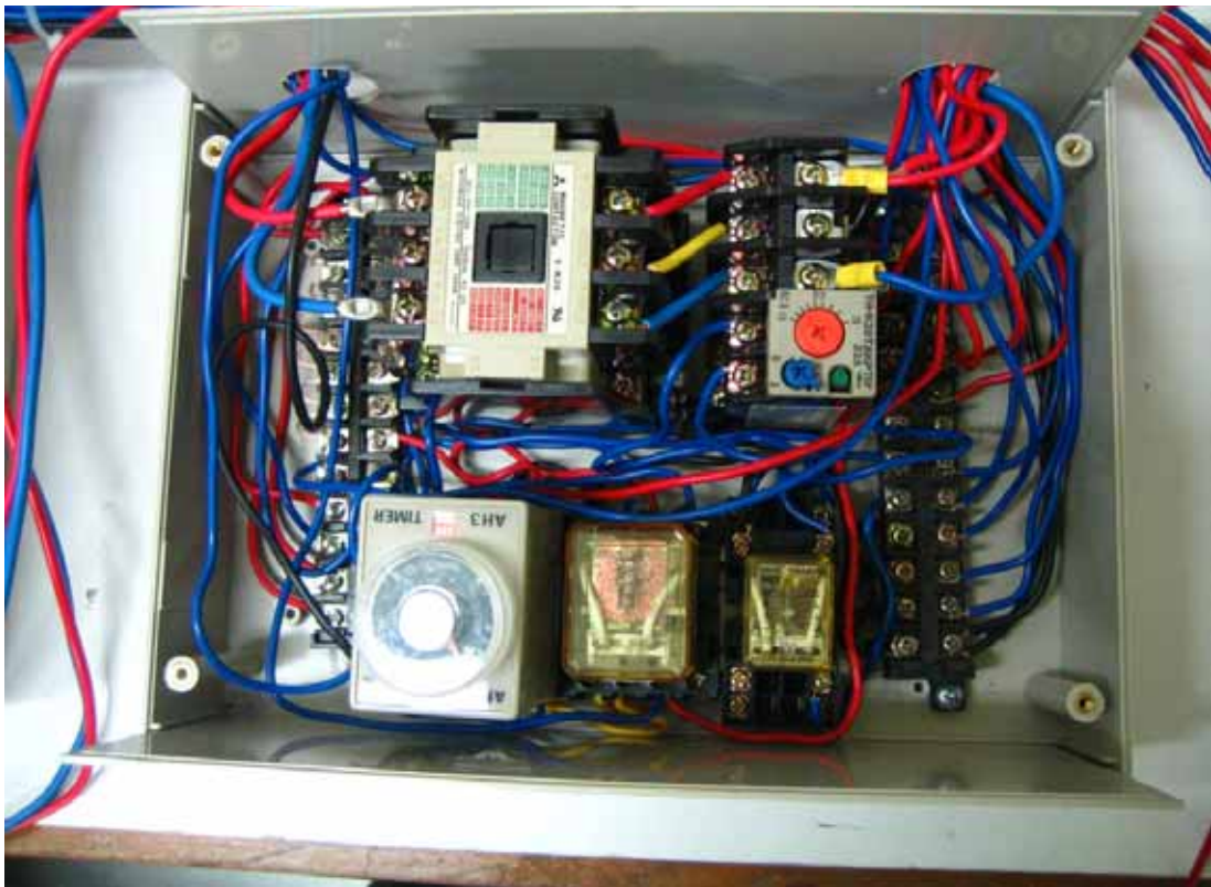
Photo 5 The data acquisition and control system
