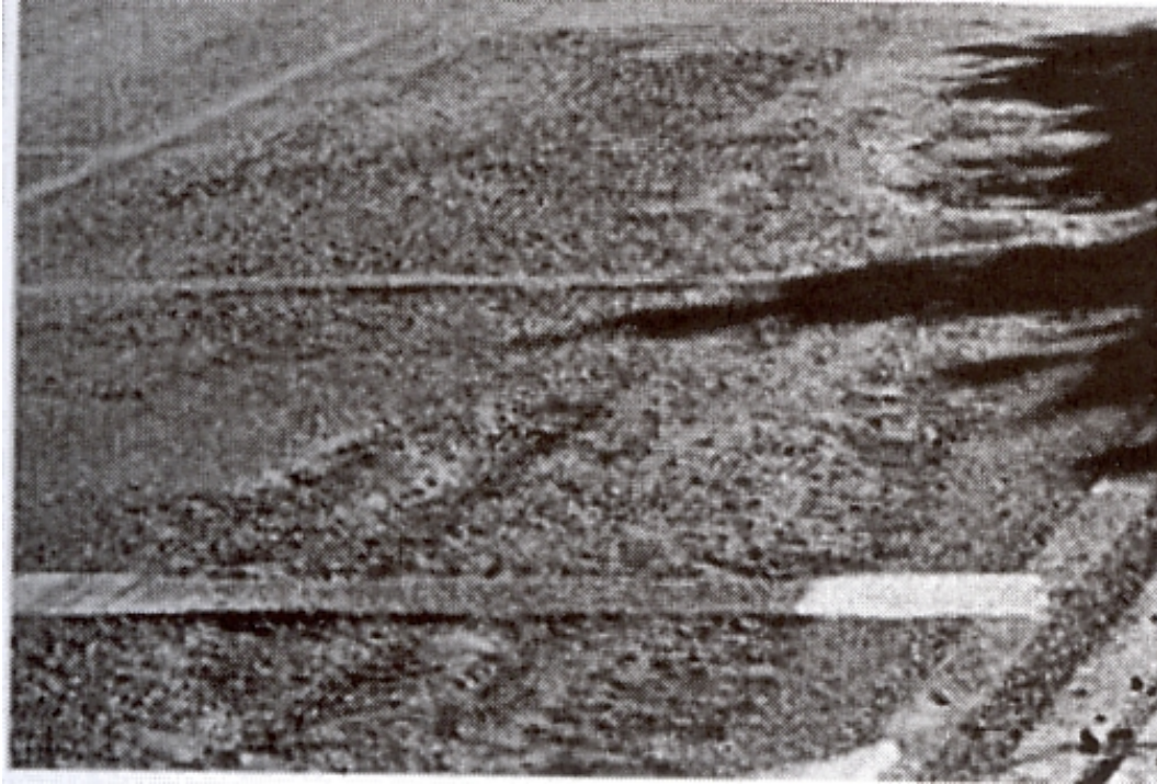
Picture 2.5 Ravelling due to Ageing and Moisture Effect
