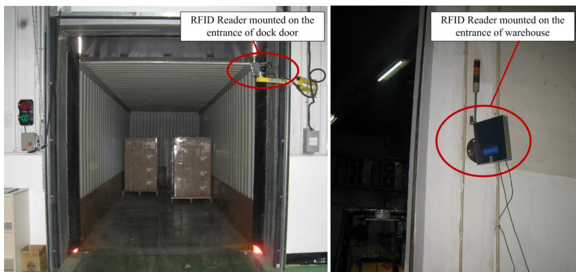
Figure 5.6 Passive RFID reader on dock door and entrance of warehouse
