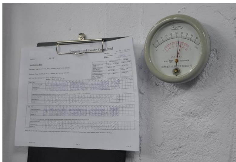
Figure 5.20 Recording temperature and humidity manually from electronic sensors
