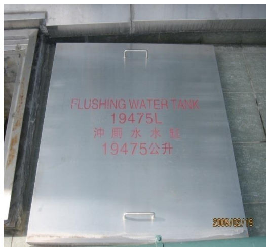
Figure 3.6 Flushing water tank (outside view)
