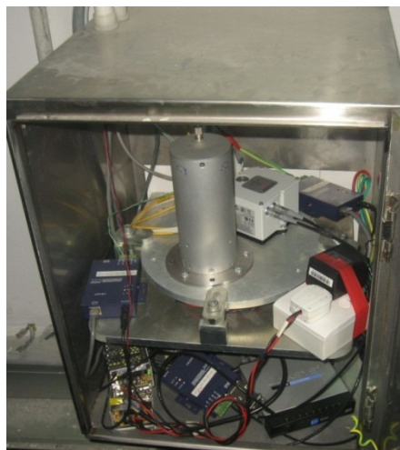
Figure 3-16. Inclinometer installed on the structure
