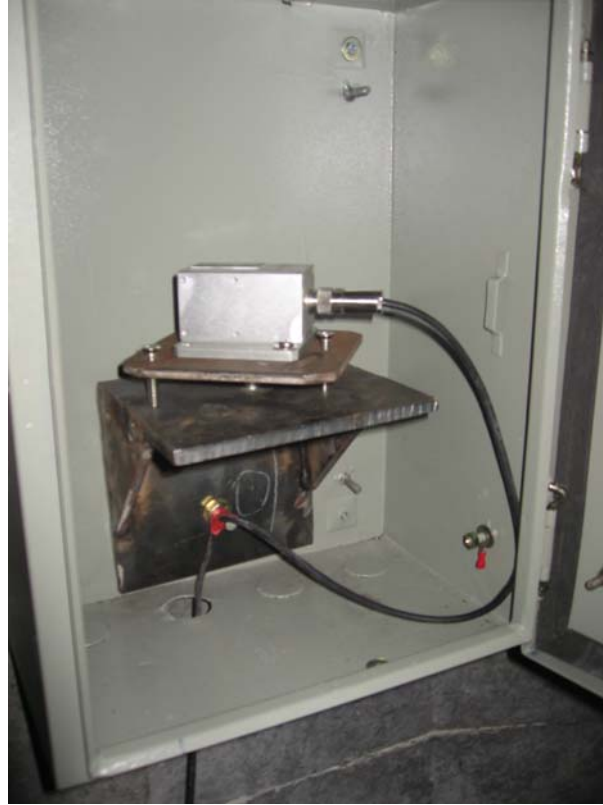
Figure 6-2. Accelerometers installed on Canton Tower
