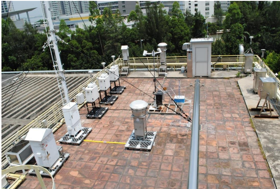
Photo 2. Tung Chung (TC) air monitoring station
