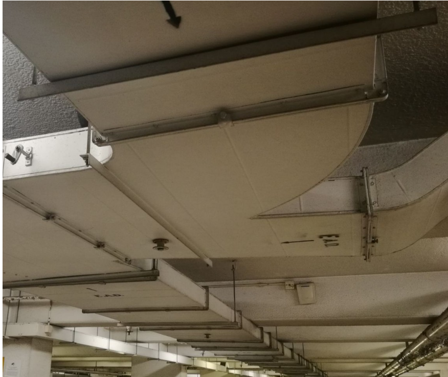
Figure 1.1: Ventilation ducts commonly found in Hong Kong.
